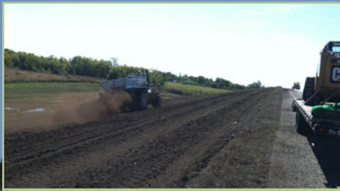
Pre-consumer-based compost was spread across the site's soil, which was first tilled one inch deep.
