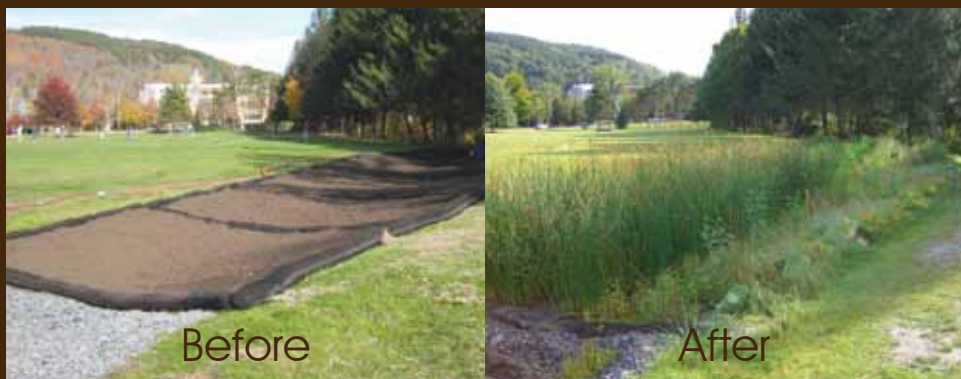
A rain garden installed 10-15-08, and the same garden less than a year later. The GardenSoxx® used on the perimeter were planted with cabbage and other edibles.
