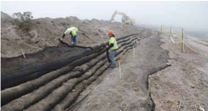
SoilSoxx at Stratford Point were filled with compost and sand, and planted with 38,000 dune grass plugs to form an artificial coastal dune system.
